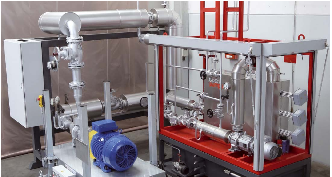
Thermal oil test stand with pump surveillance system on the premises of Speck in Roth. Research of impacts of high temperatures up to 350 °C on the lifetime of the pumps.
